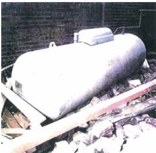
Figure 21 – The one-tonne storage tank
