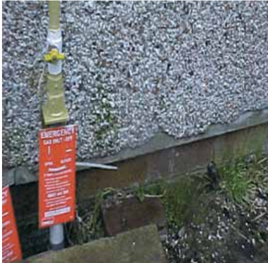
Figure 15 – Typical Emergency Control Valve (ECV) on outside of property
