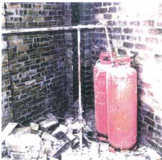
Figure 22 – The two manifolded 47kg propane cylinders
