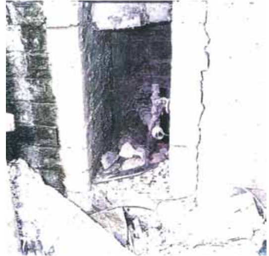
Figure 24 – The LPG underground pipeline enters the building in an alcove in the basement
